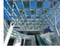
Building-integrated photovoltaic (BIPV) modules
