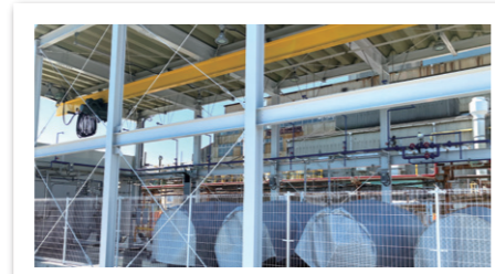
Storage tank for ammonia fuel
