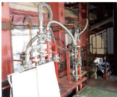
Glass melting furnace in which this demonstration test was conducted
