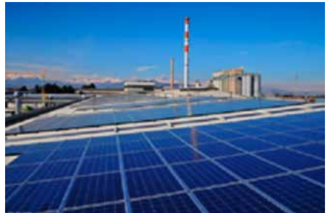
Photovoltaic panels at the Cuneo Plant (Italy)
