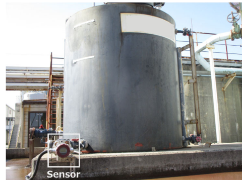
Tank inventory management system
