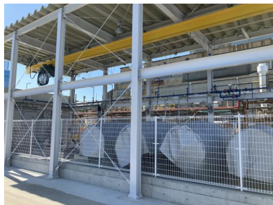
Storage tank for ammonia fuel
