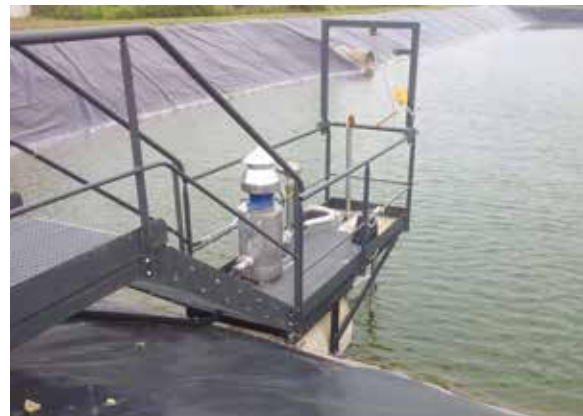
Storm water recovery system in Seingbouse, France.
