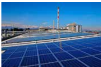
Photovoltaic panels at the Cuneo Plant (Italy)
