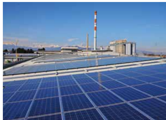
Photovoltaic panels at the AGC Flat Glass Italy
