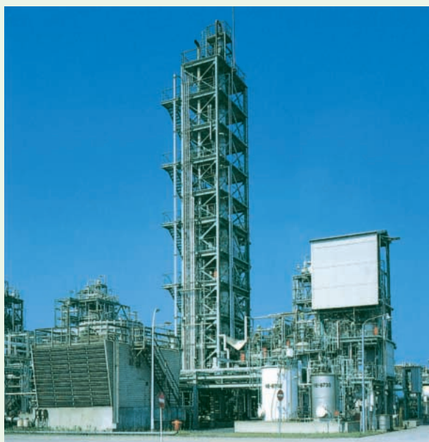
Fluorocarbon resin facility, one of the facilities recognized resistered high-pressure gas
