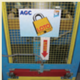
A sign indicating a Lock-Out location
