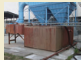
Tank for wastewater reuse
