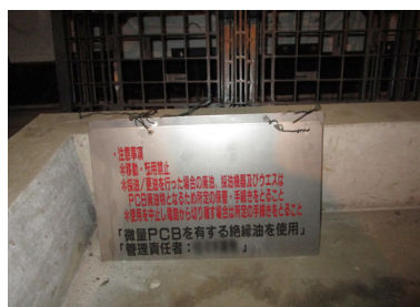
Storage area for low-concentration PCBs (Sagami Plant)
