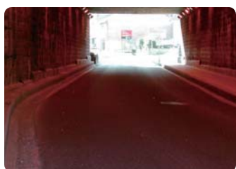
A practical test in Belgium, with the reflecting road surface being used in a poorly illuminated tunnel
