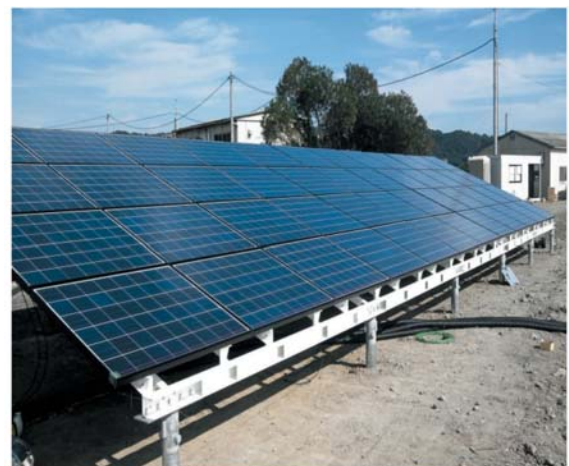
Fig.10 GFRP frame of the solar module for the experimental facilities in Setouchi.
